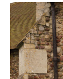
9.3.2 Repoint north east buttress to North aisle on west side at high level 14.4 £300
